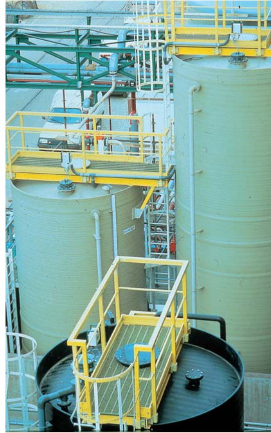
Liquid storage tanks with Allgrid flooring : 100% resistant to corrosion. (Allgrid on page 95).
